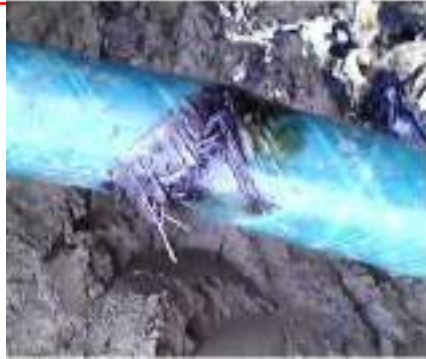
Pipe body fracture
